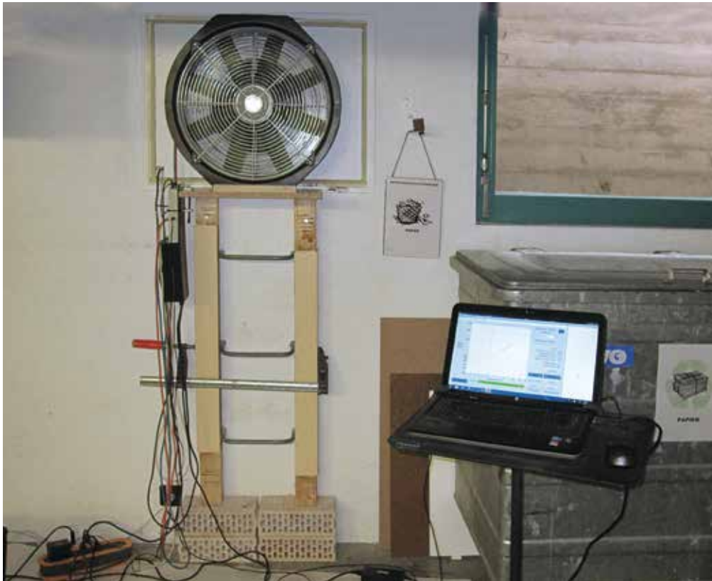
Figura 6.49: Test blower door.
